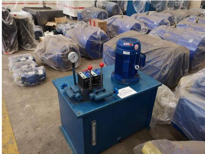
hydraulic oil station
