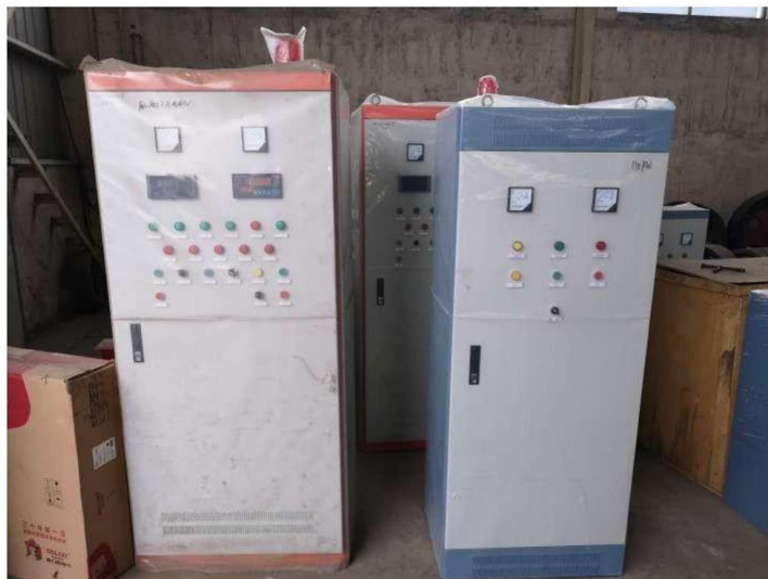
Electric control cabinet
